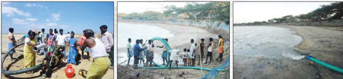
Installation of diesel pump and laying pipe line to provide seawater supply to the pond
