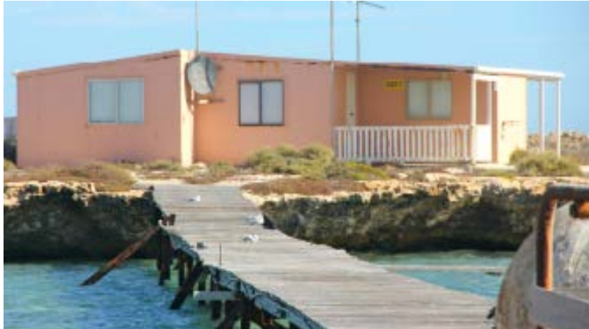
Closed and decaying infrastructure on the Houtman Abrolhos islands, Australia, following fishery management and climate changes that have more recently lacked full community consultation and excluded women’s views. Source: Jenny Shaw and Leonie Noble
